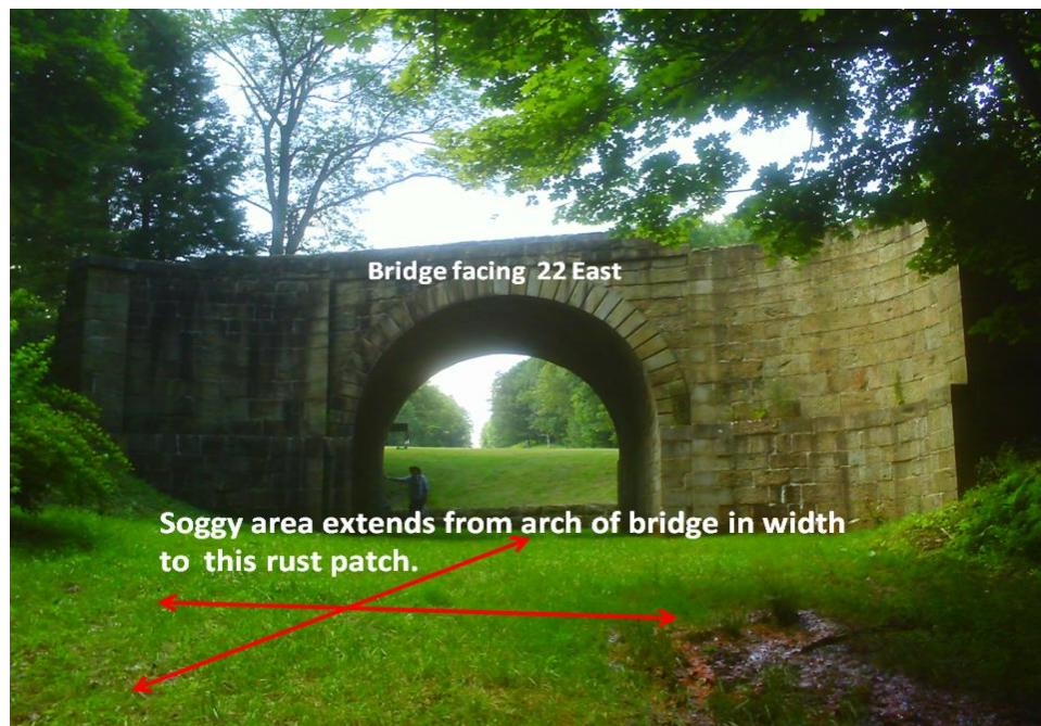
Figure 12: Image of evaluation of grounds in the immediate area of the Skew Arch Bridge.
