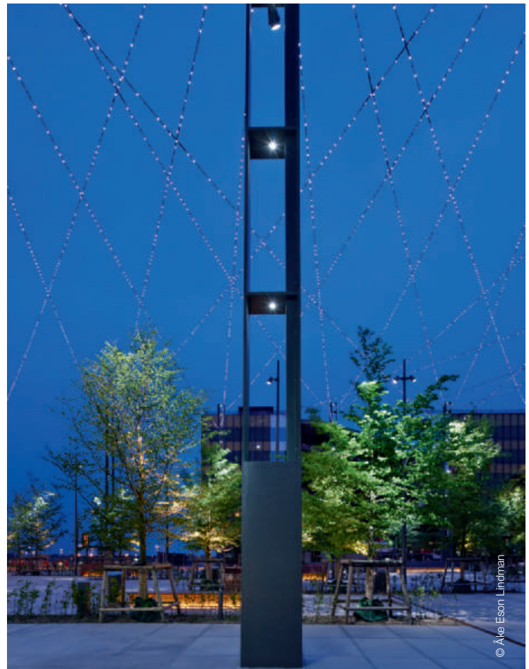
Bases of the transparent masts in which the floodlights are fixed, with wires above.
