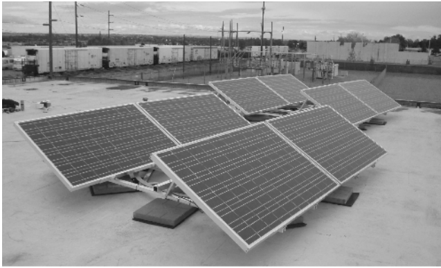
Figure 1.2. Two-kilowatt PV array from JX Crystals Inc on a commercial building flat rooftop.
