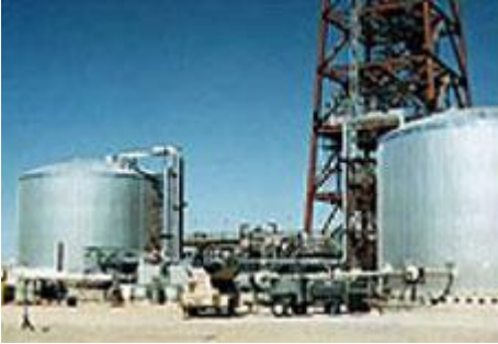
The two-tank direct molten-salt thermal energy storage system at the Solar Two power plant.
