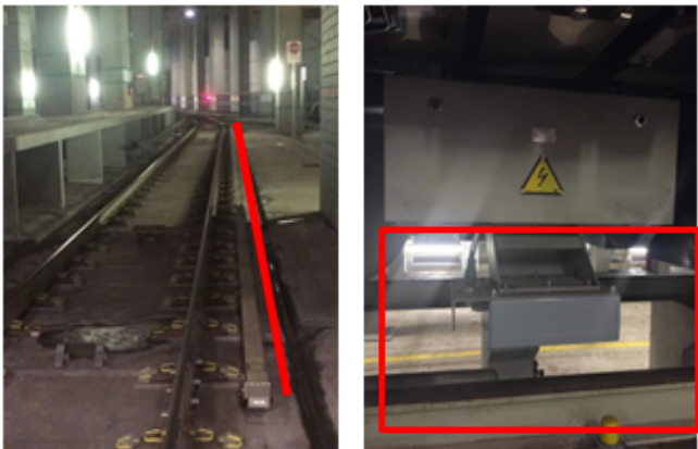
Fig. 1. Leaky waveguide deployment in railway systems (left) and the corresponding trainborne antenna (right)
